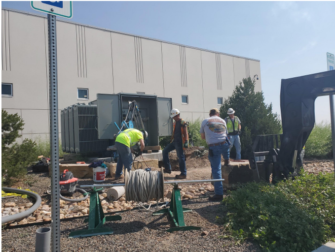
New 3MW Transformer - Contracting Team is pulling the 24.9kV cables in place - July '21
