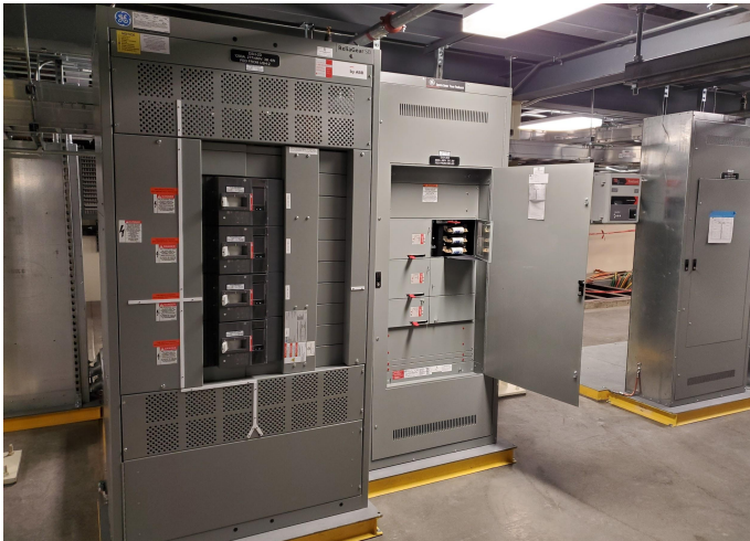
480v Distribution and Fuse Board Panel associated with Derecho Compute Nodes
